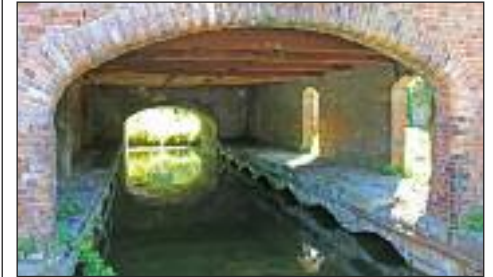
The Transhipment Warehouse over an arm of the Newport Canal Photo: © Andrew Tidy
