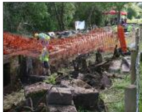
In the foreground is some of the ironwork from the decayed lock gates
