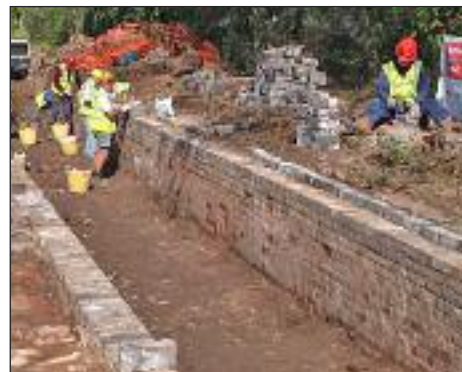
Work starts on laying the bricks salvaged from work around Lock 20 (Newport Town Lock)
