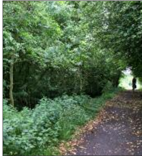
The canal and towpath prior to restoration showing the amount of vegetation that had to be removed from the bed of the canal
