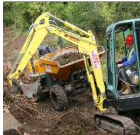
A mini-digger and dumper truck were employed to move the tons of earth and stone used to fill the lock
