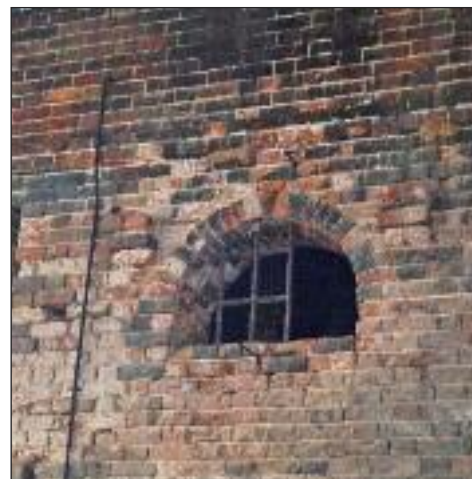
Bricks are removed from one of the bricked up windows in the Transshipment Warehouse
