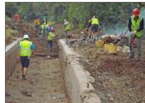
The bricks have been laid and covered to dry, while the team tidy the site ready for grass seed to be sown
