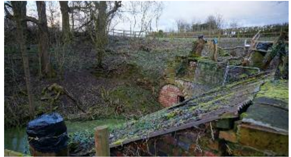
View of the tunnel entrance from above with the new fence in place
