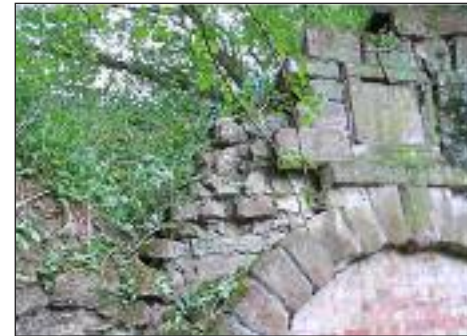
Damage to the portal masonry
