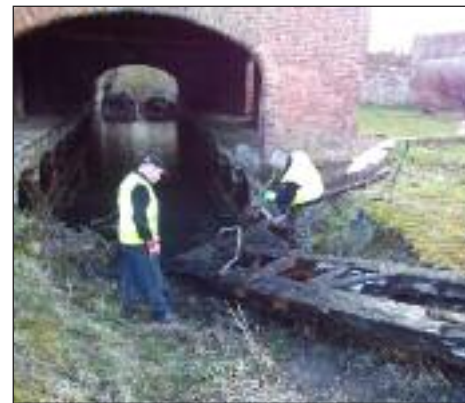
Phil with the old stop gate after being pulled from the water
