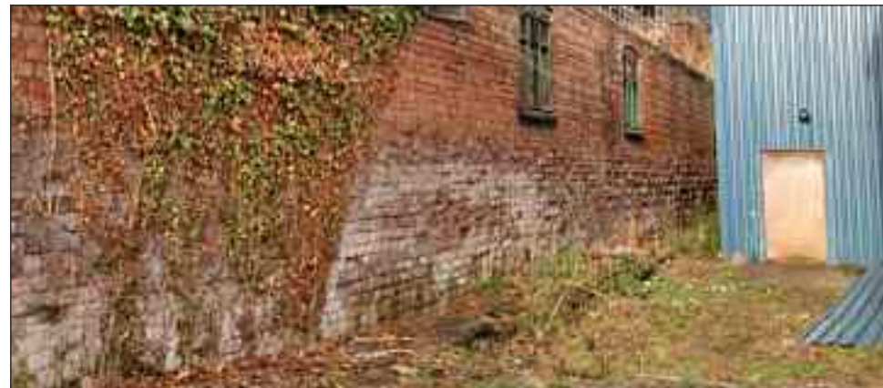
Shrewsbury Canal stone edge coping just visible (adjacent to brick wall) at Ditherington Flax Mill Maltings
